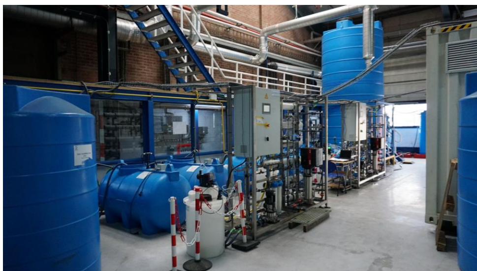
Site II Build-up at Plant One in Rotterdam. Image: ZERO BRINE
